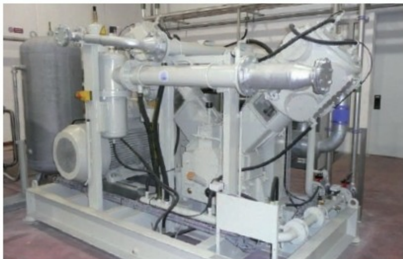
Leak prevention system (LPS) on a skid
