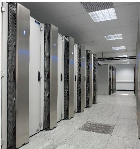
ColdLogik CL20 rear cooler solution
